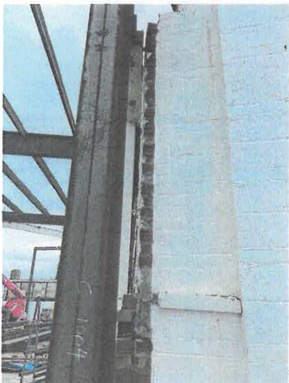
Photo shows gap between wall and existing columns
