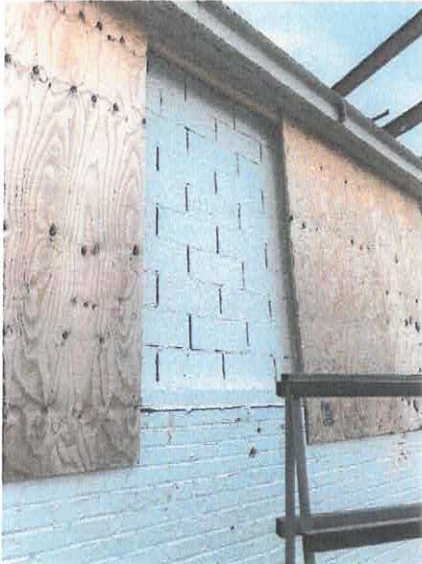
Photo shows top course of brick crack at joint
