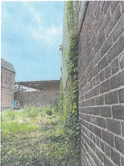
Photo taken from exterior shows leaning wall above
