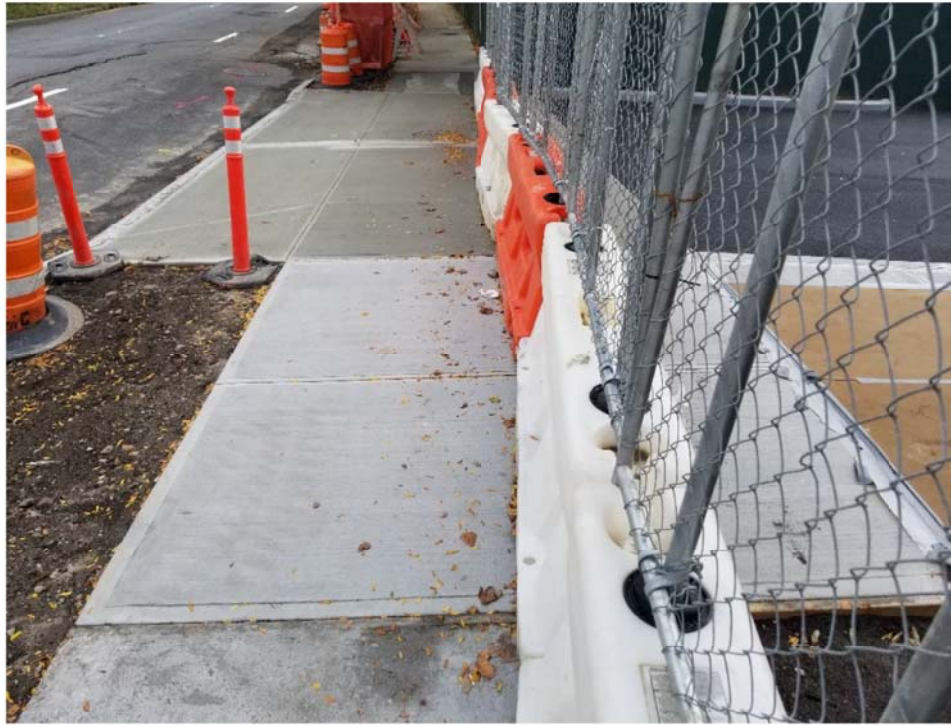
Photo 1 Curb Cut – looking East on Horace Harding Expressway
