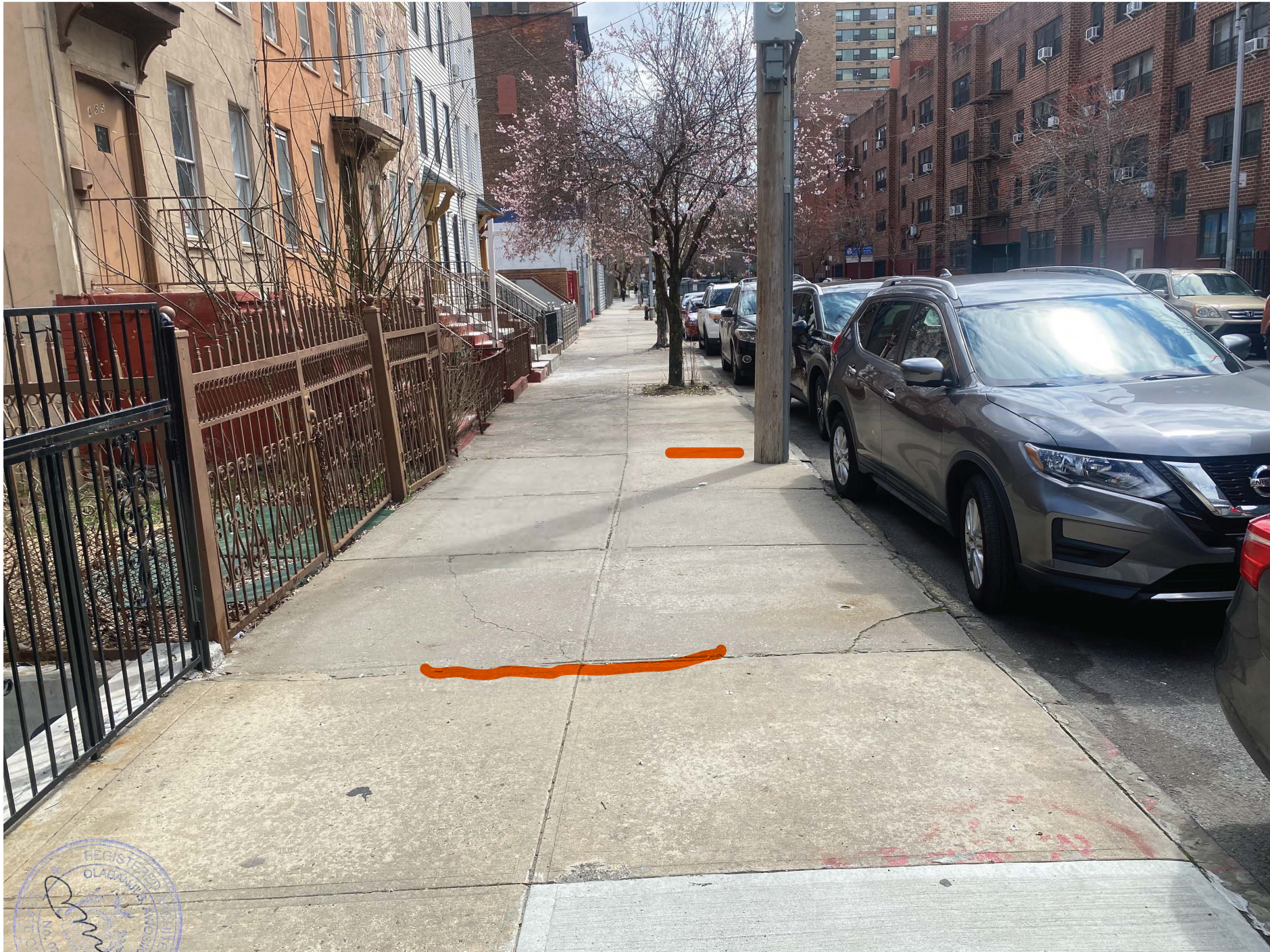
PHOTO SIDEWALK 2 463 EAST 143 STREET, BRONX
