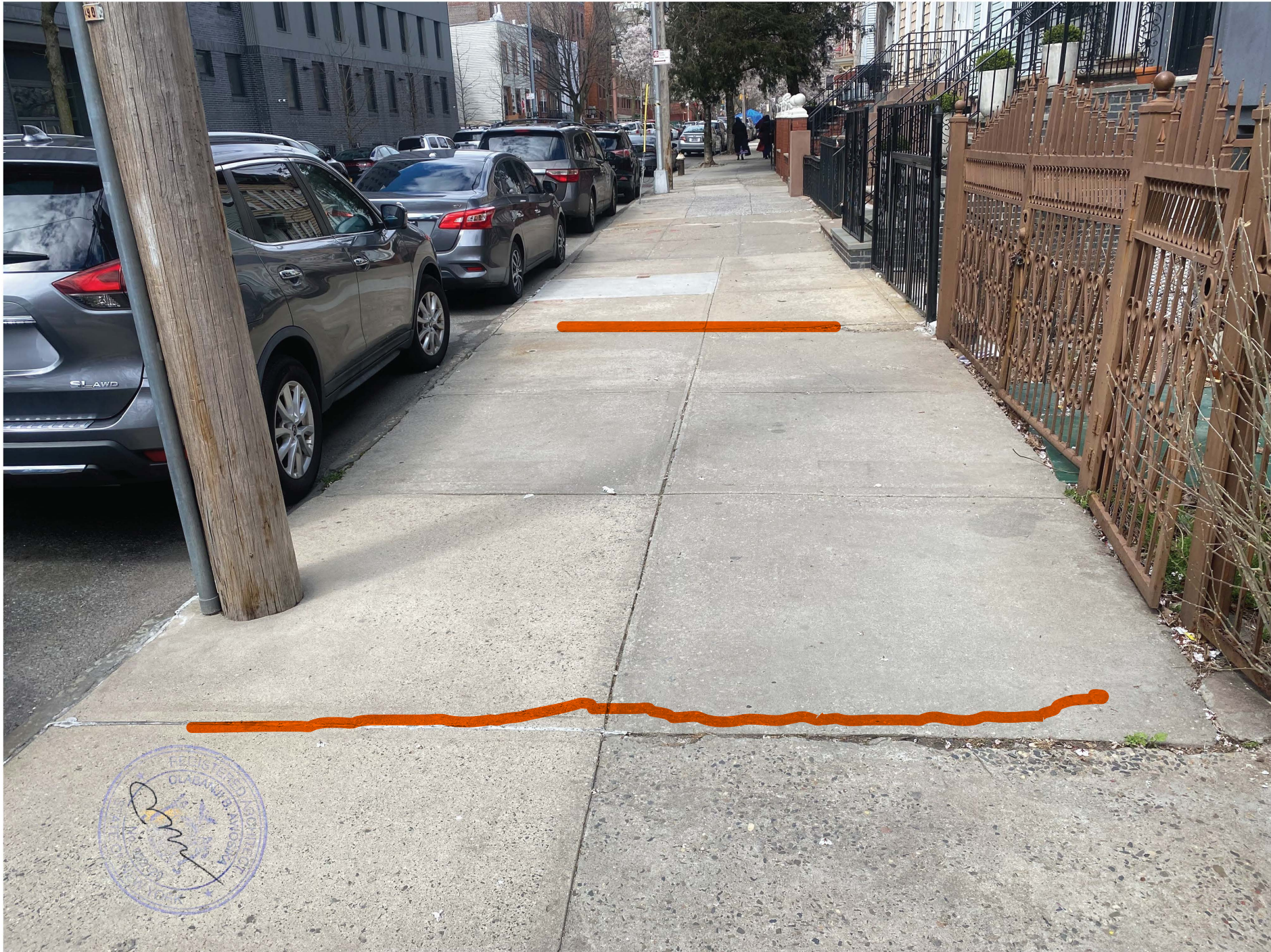
PHOTO SIDEWALK 1 463 EAST 143 STREET, BRONX
